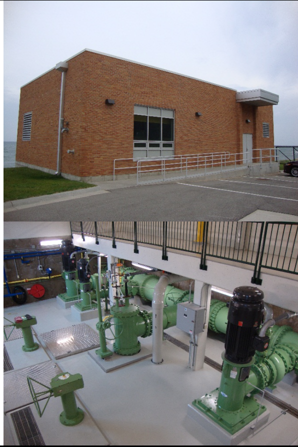
North Low Lift Pump Station
