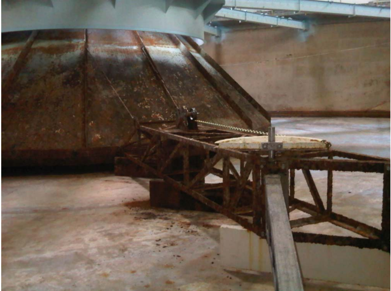
Solids Contact Clarifier No. 2 Dewatered
