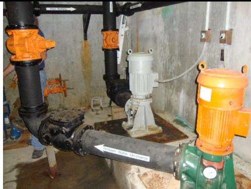
Filter Backwash Recycle Pumps
