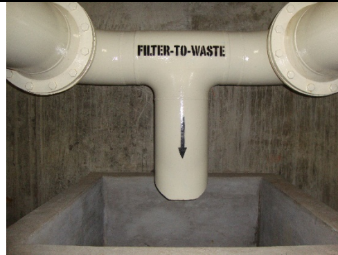
Filter #11 and #12 Filter-to-Waste Lines
