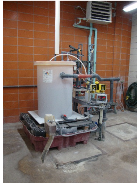
Day Tank and Metering Pumps
