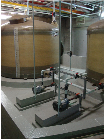
Bulk Storage Tanks and Transfer Pumps
