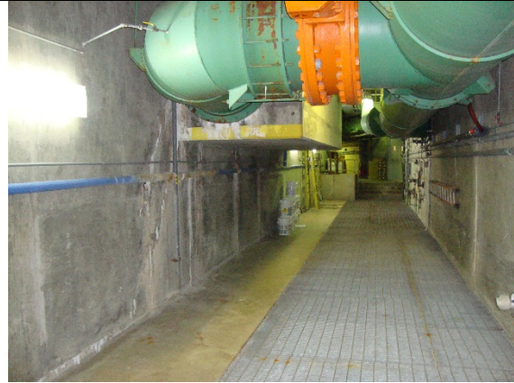
Clarifer #2 and #3 Settled Water Pipe Gallery
