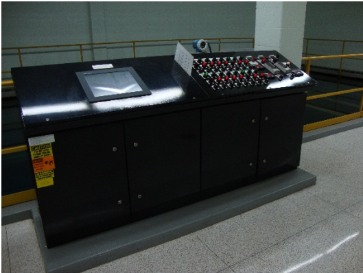
Filter #11 and #12 Control Console
