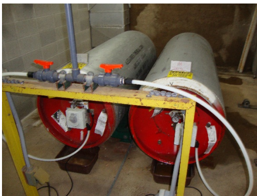
Gas chlorine 1-ton cylinders
