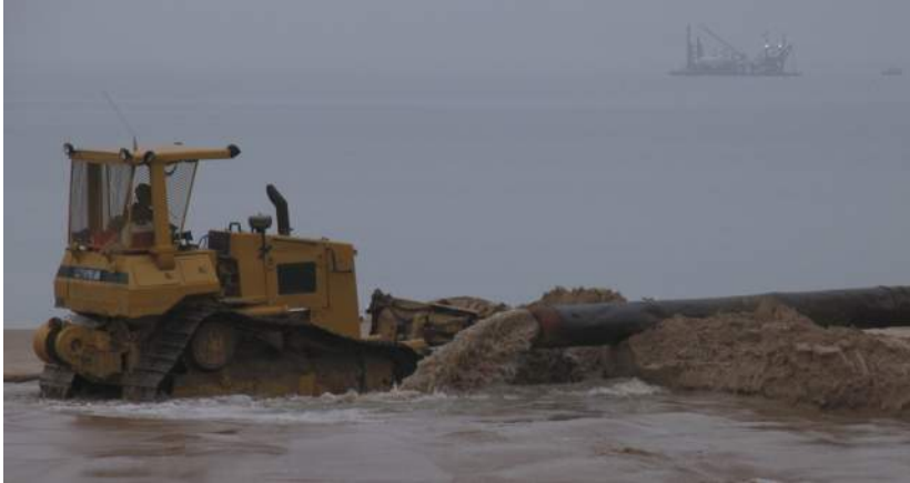
Figure 18: 2012 photo of beach nourishment south of Park Street showing the dredge in background
