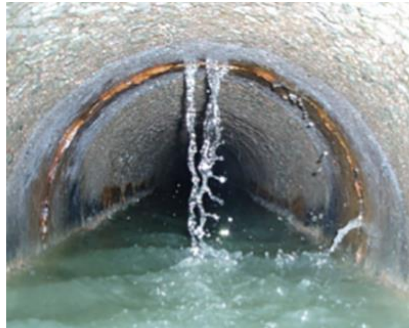
Example of infiltration in a sewer pipe
