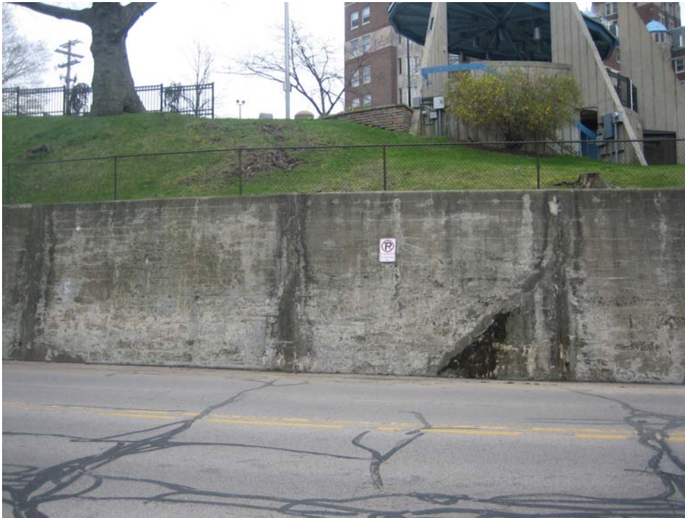
PHOTO NO. 33: Note the cracking and concrete deterioration in the retaining wall.
