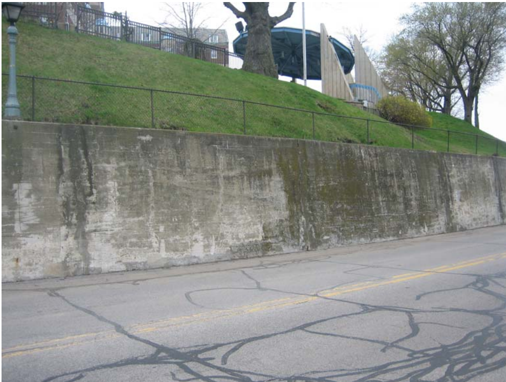
PHOTO NO. 34: Looking southwest at the concrete retaining wall along Water Street.
