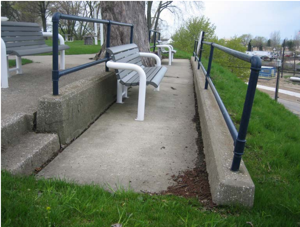
PHOTO NO. 29: Note the lean (downslope) in the wall and handrail at right.
