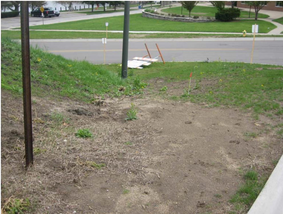
PHOTO NO. 37: Erosion due to concentrated surface drainage.
