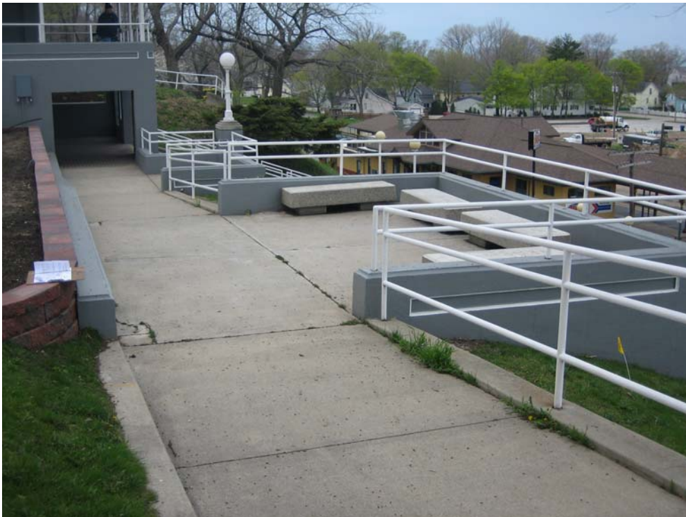
PHOTO NO. 26: Surface drainage from flatwork is being discharged onto the bluff face through scuppers in the walls.
