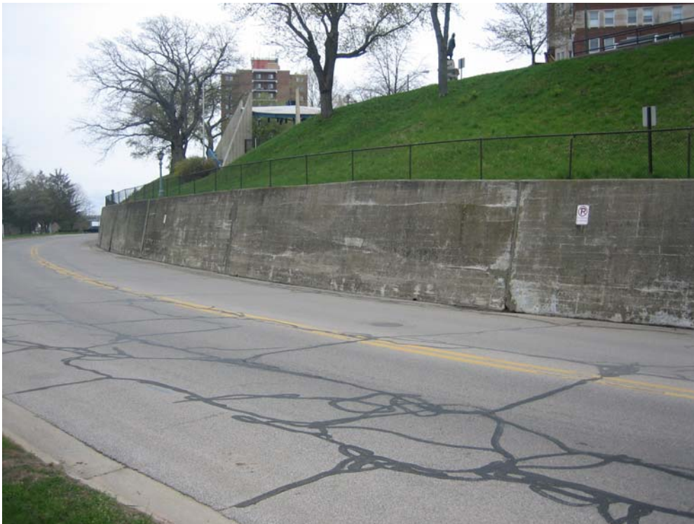
PHOTO NO. 30: Concrete retaining wall along Water Street. Note cracks in the concrete.
