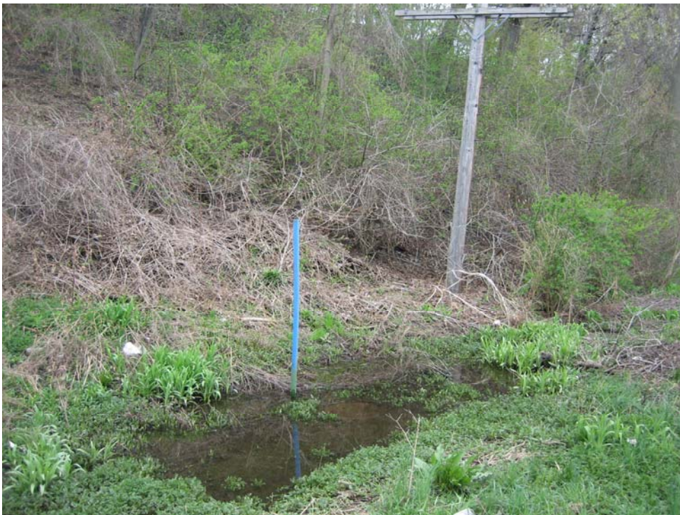
PHOTO NO. 12: Wet area at toe of bluff likely due to poor surface drainage.
