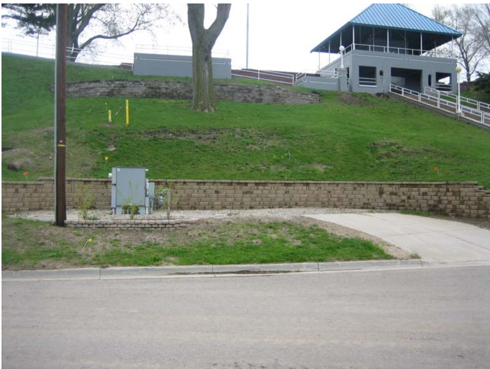
PHOTO NO. 24: Looking southeast. The lower MSE wall is in good condition. The upper MSE wall (behind the tree) is experiencing excessive deflections at the top.
