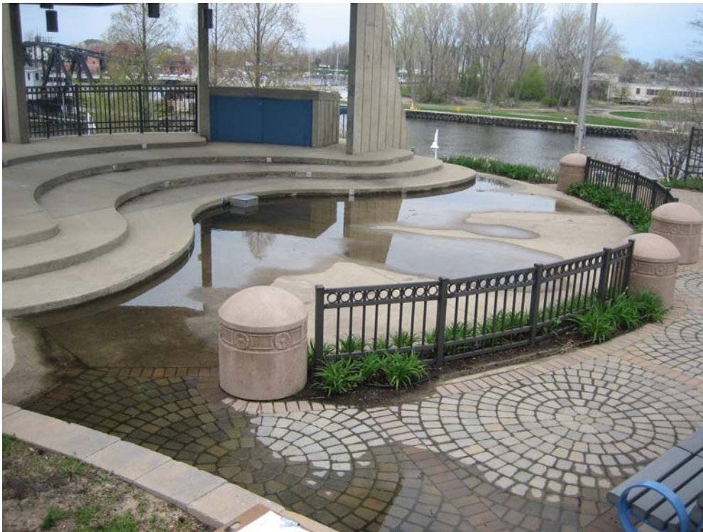
PHOTO NO. 38: Ponded water in the flatwork area of the Howard band shell.
